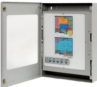
View showing mimic mounted on inner door
